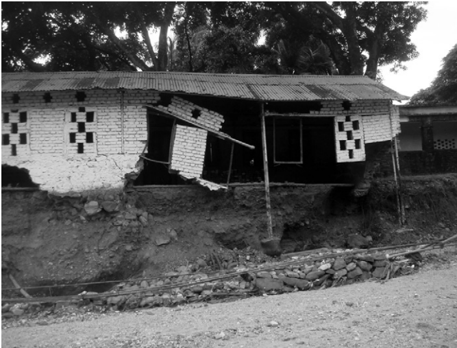
Fig. 2. Destroyed School Building After a September 2009 Flash Flood, Khahare Khola. Photo: Dubois (2009).
